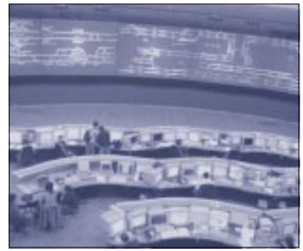
The Operations Control Centre (OCC) at Tsing Yi MTR Station
